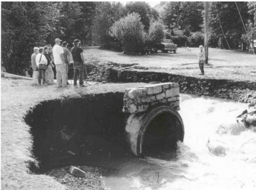
Hazard Mitigation Grant application submitted to assist 7 households repeatedly flooded by Shoups Run and Sugar Camp Run in Carbon Township
